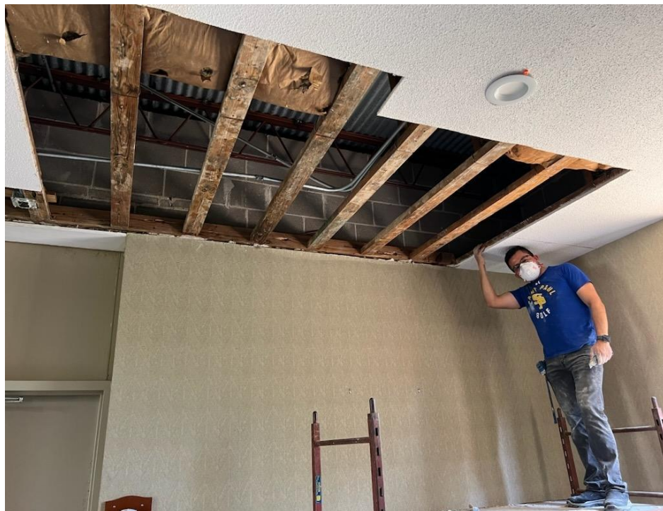
St. Paul's Maintenance Crew repairing ceiling damage from a recent roof leak at Our Lady of Peace Student Chapel.
